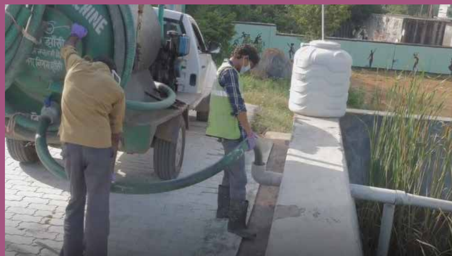
Sludge being fed into the Planted drying beds
