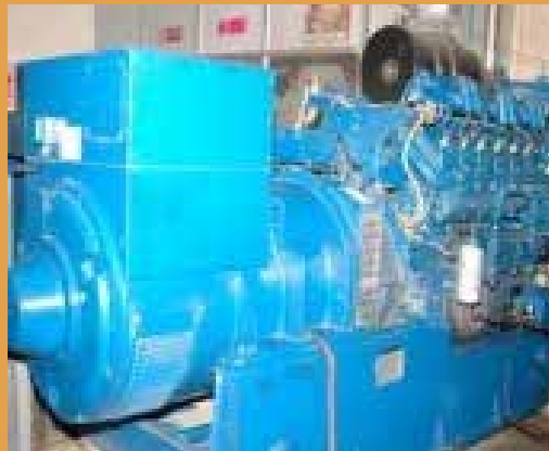
Biogas engine for power generation, Nessapakkam STP
