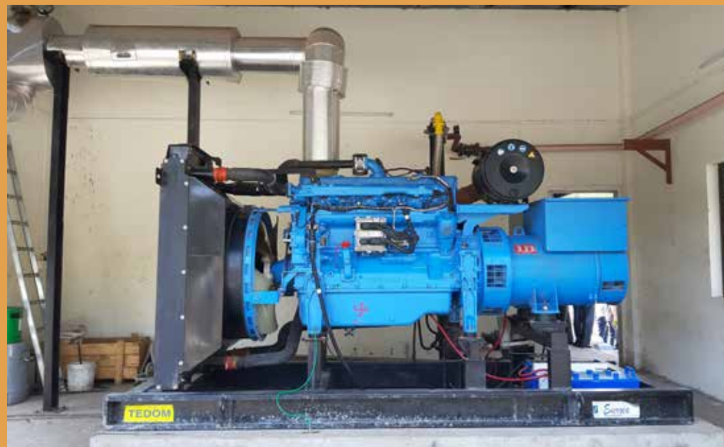
Electricity Generator at Biomethanation Plant
