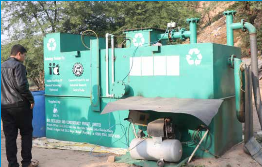
Biogas plant at Nada Sahib Gurudwara
