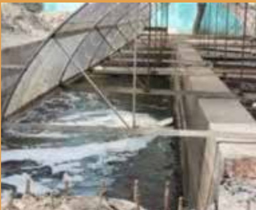
Receiving Tank- Decanting Station Source: https://www.cseindia.org/nesapakkam-stp-chennai-8642
