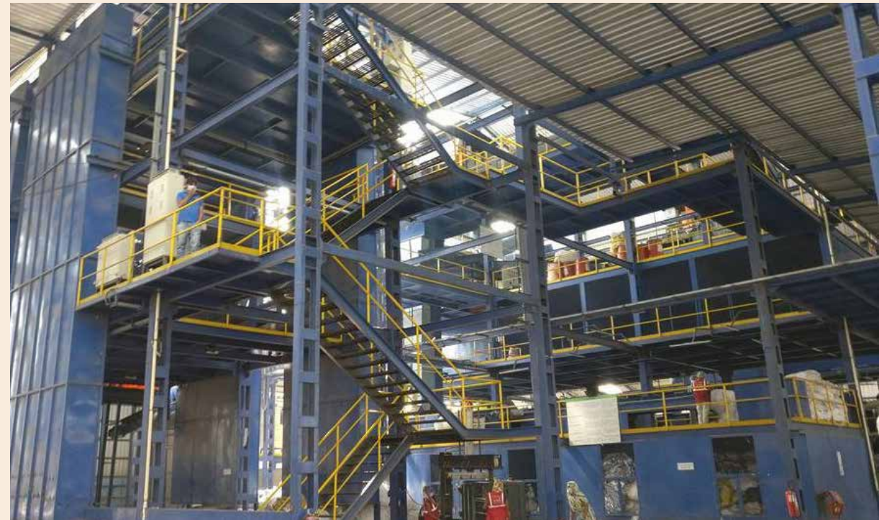
Material Recovery Facility- NEPRA, Ahmedabad
