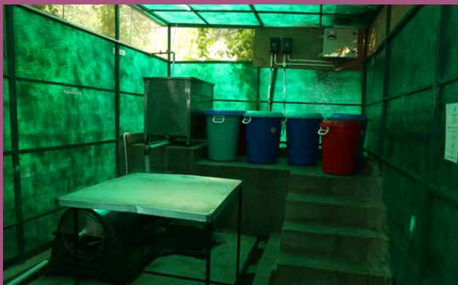
Space allocated for collection and processing of segregated waste at Silver Oak
