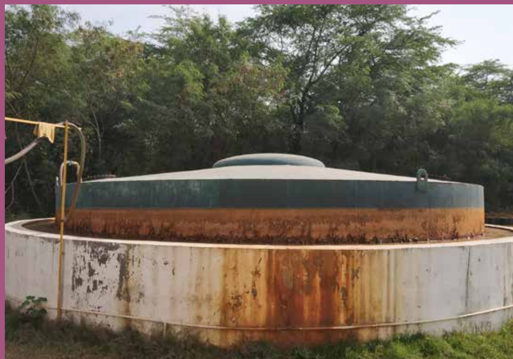
Bio-Methanation-Cum Electricity Generation Plant
