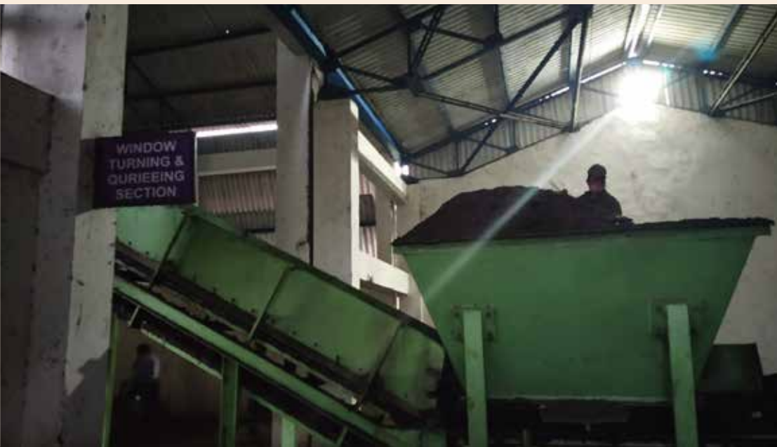
Mechanical composting plant at Moshi
