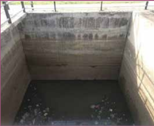
The Storage Tank
