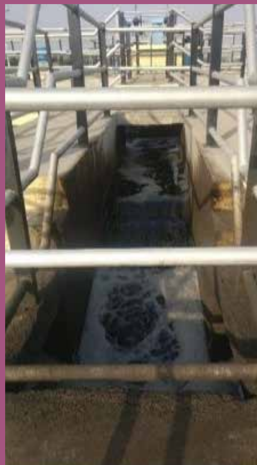
Pumping after screening
