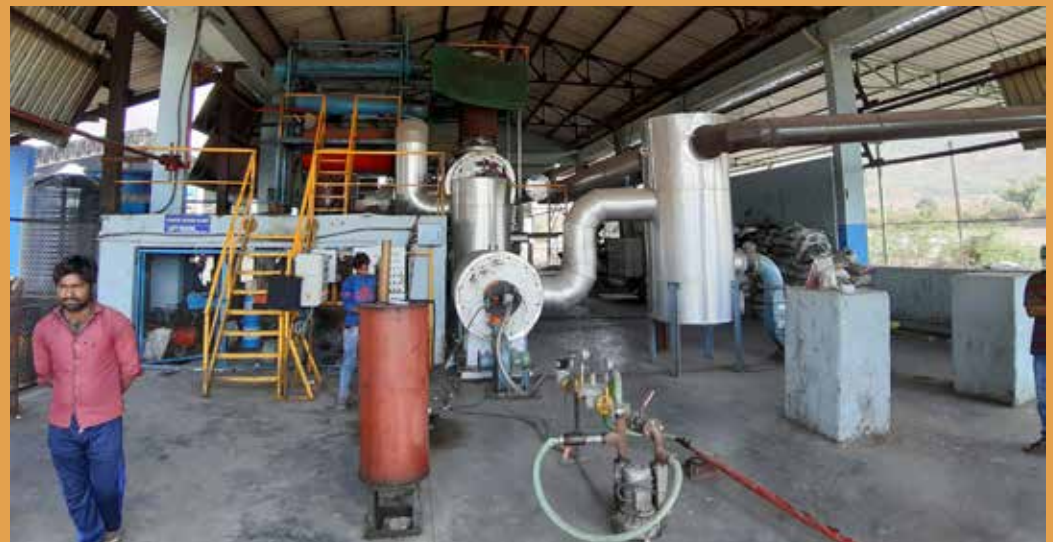
Plastic to fuel plant
