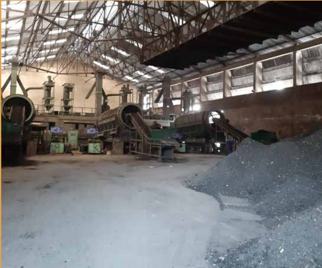
Trommels in composting plant
