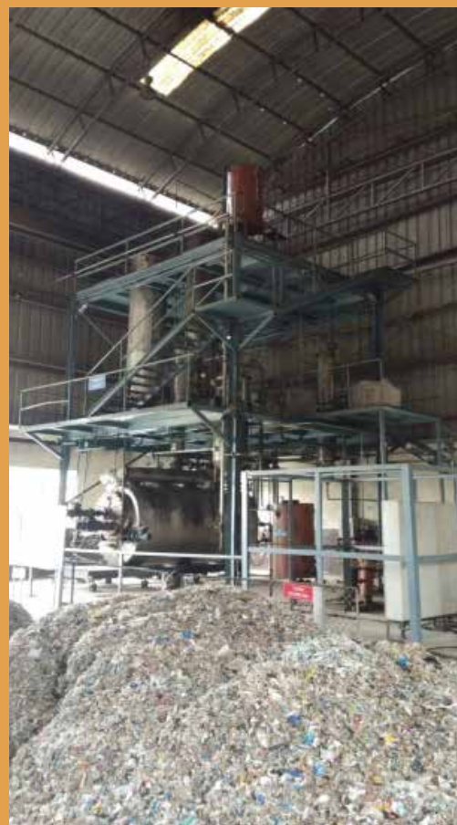
Plastic to fuel plant
