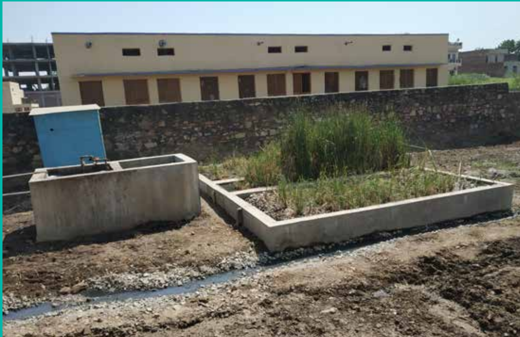
Drainage Treatment Plant
