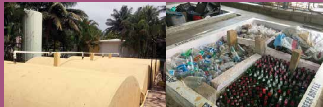
Biogas facility at Infosys Campus, Mysore
