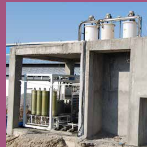
Leachate Treatment Plant
