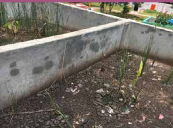
Planted drying bed, FSTP
